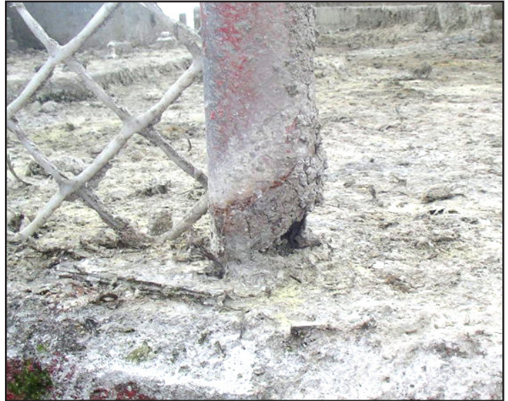
Bird feces corrodes a metal post
